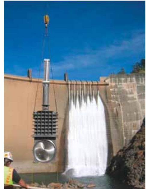
78" Hydro Guard Valve, 130 psi, CS with 304 SS Trim, For Fixed Cone Valve Isolation, Englebright Dam, California
