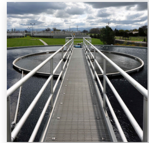
Potable Water Treatment
