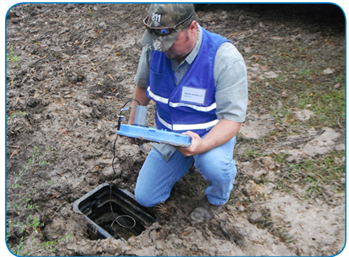
Michael Guimbellot, distribution, installs an ORION Cellular endpoint as part of the BEACON AMA managed solution.
